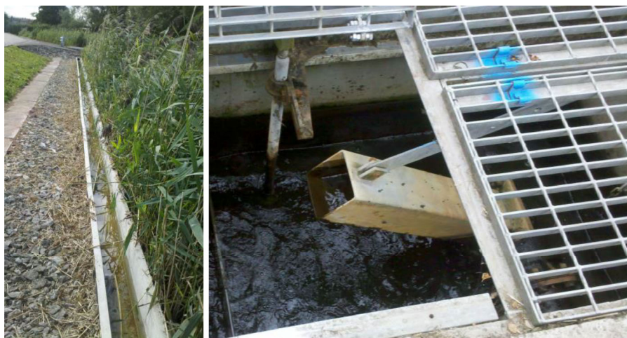
Figure 3.2 Examples of civil structures in HF wetlands; left: distribution troughs; right: water level control structure.
